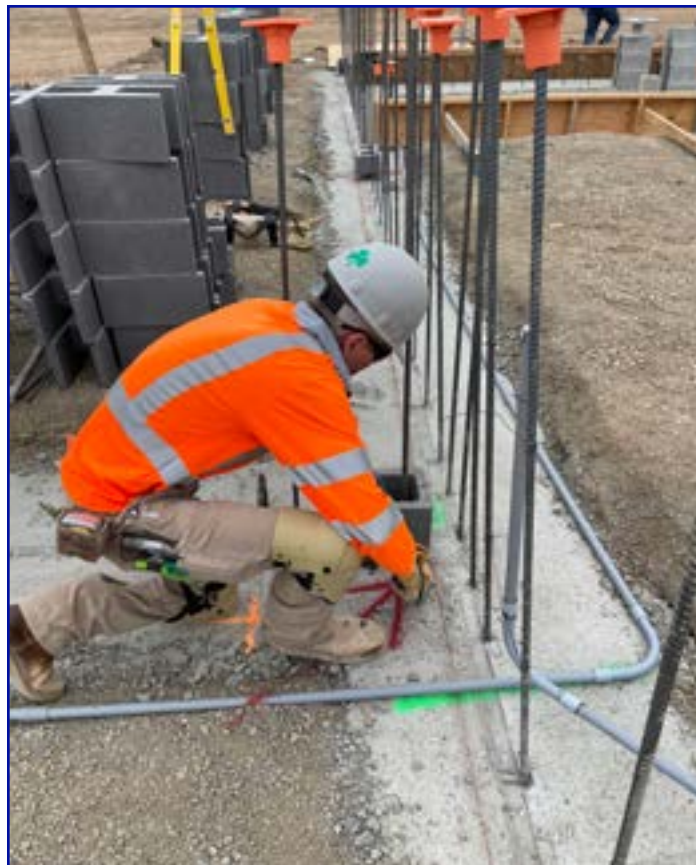
Paul McCloskey Laying the first course of block at the Napa County Jail with Bratton Masonry.
