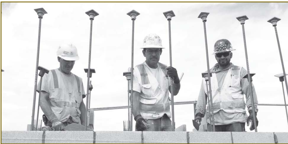
L to R: Ramo Ruznic, Miguel Montano and Eddie Aguilar / Cornerstone Masonry
